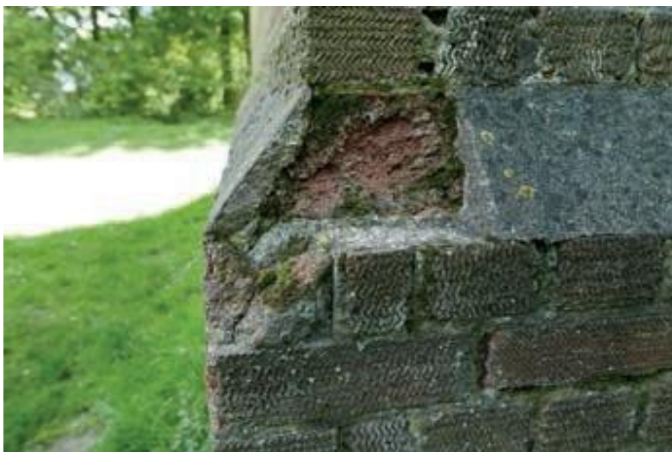
Figure 8 Detail of damage to plinth
