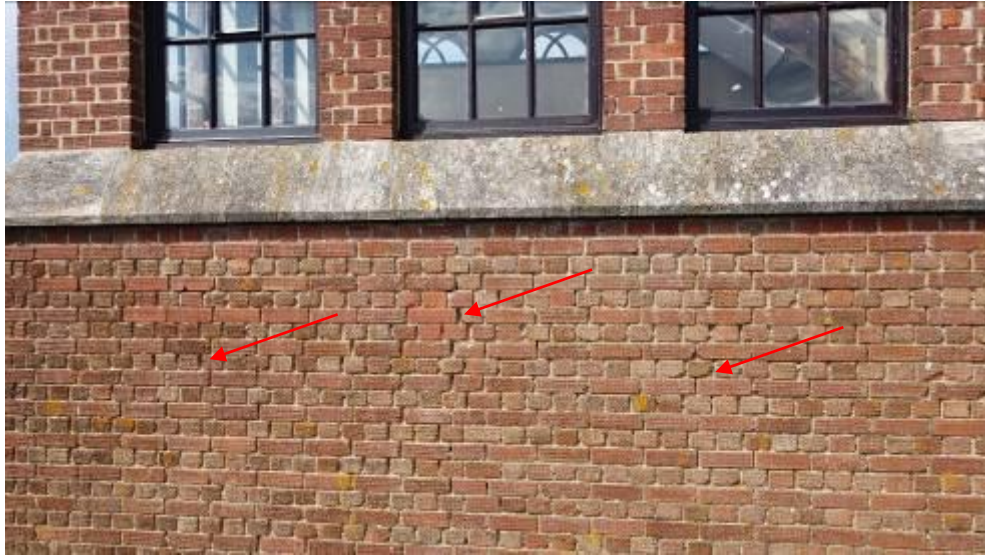
Figure 5 Cill/string course below windows in south wall of Belvedere showing deep open joints in brickwork
