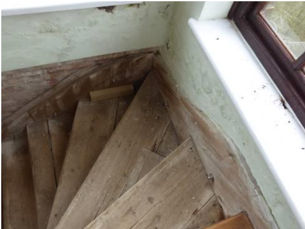
Figure 18 Detail of same with corresponding decay in stair joinery
