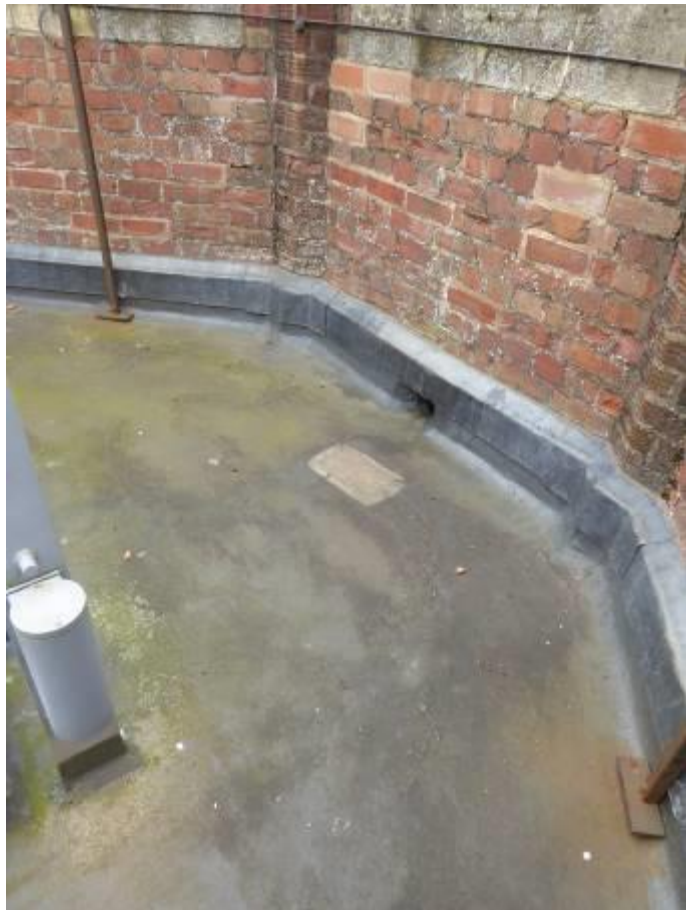
Figure 9 General view of north side of roof with asphalt covering and lead cover flashings
