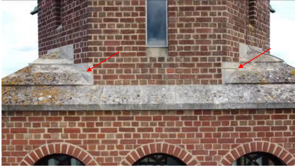
Figure 3 Erosion to stone 'broaches' at south-west and north-west corners between Lantern and Belvedere rooms
