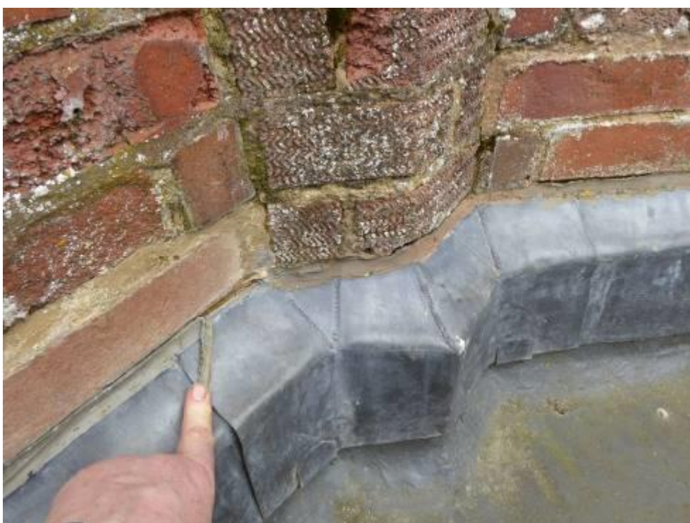
Figure 12 Silicone mastic removed at head of lead cover flashings reveals shallow section of lead in rebate in brickwork
