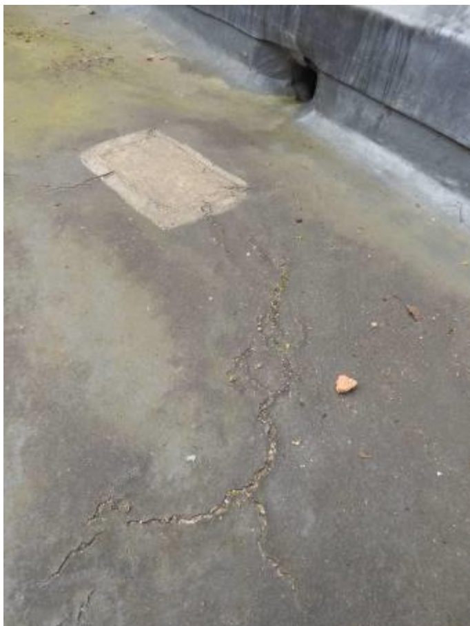
Figure 10 Detail of same showing patch repair and cracking to upper surface
