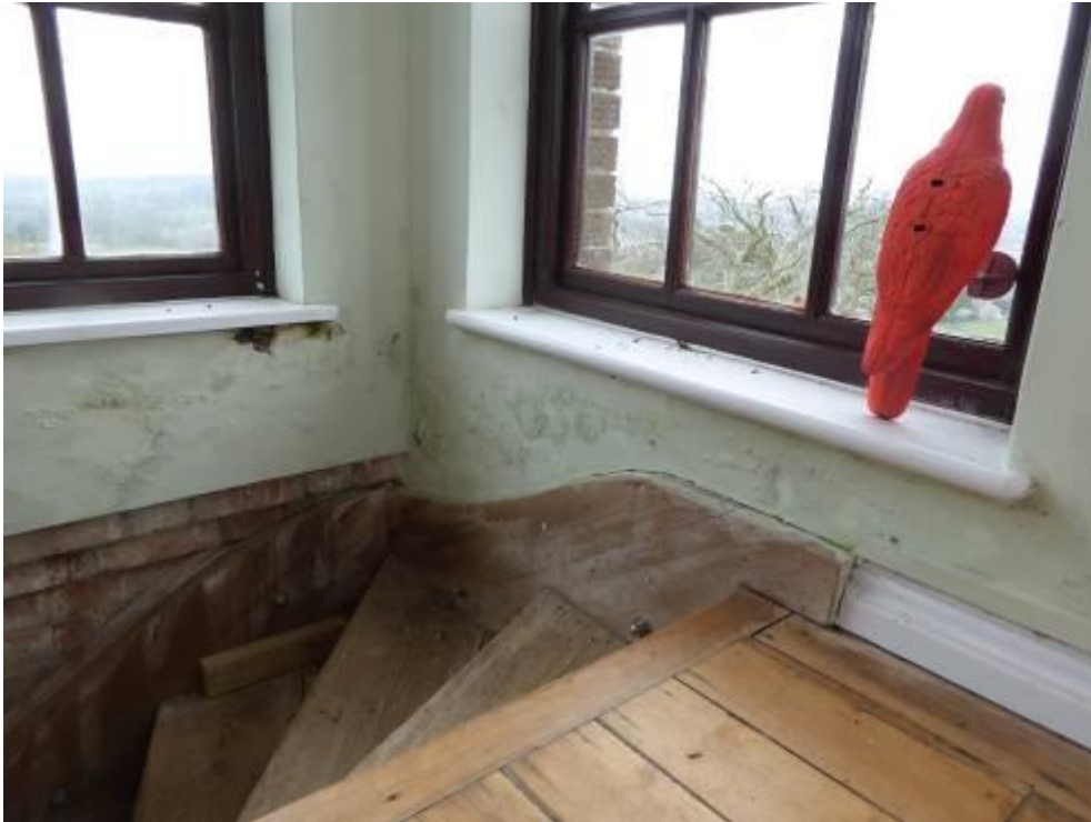
Figure 17 Damage to internal wall finishes in south-west corner of Belvedere room – this occurs generally on the weather sides and appears to be due to failure of pointing between the timber window cills and stone cills below
