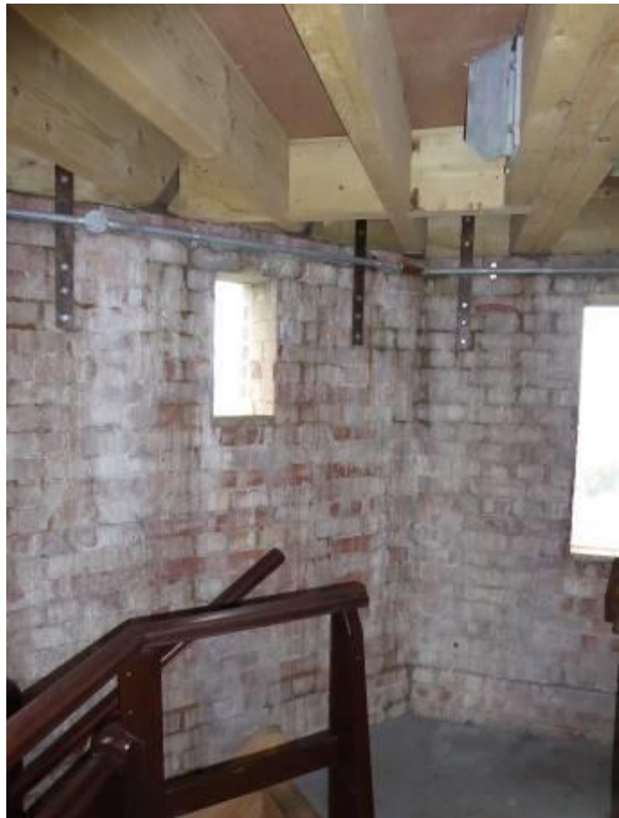
Figure 15 General view of south and west walls of Lantern room with signs of recent water ingress
