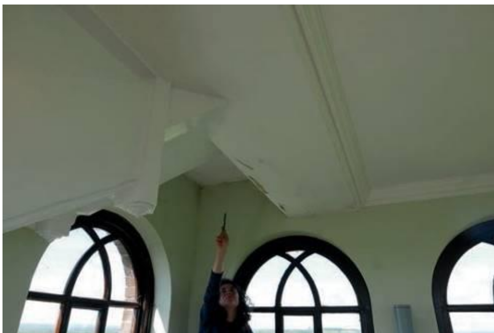
Figure 19 Mould growth and disruption of decorative finishes to west end of enclosed trimmer beam to ceiling of Belvedere room
