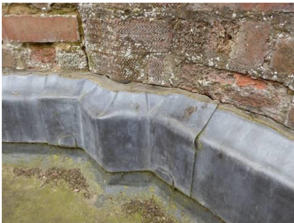
Figure 11 Open joint at head of lead cover flashing to roof
